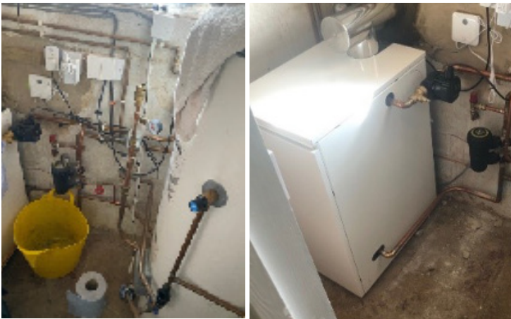
The Sapphire boiler finished and commissioned.
